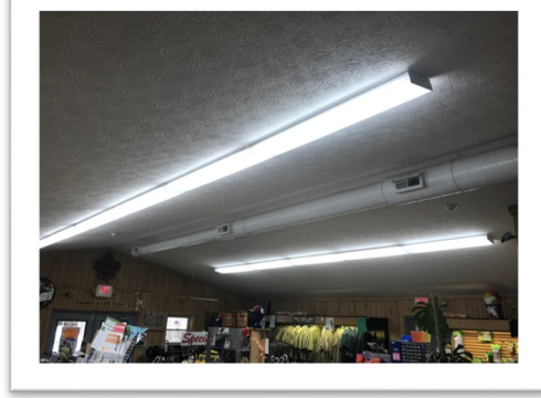
LED Lighting for Camp Store & Campmaster Cabin
