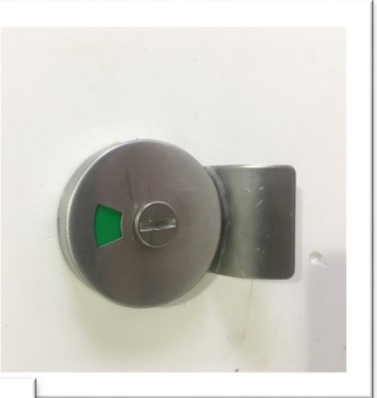
Door Latches for Wyandot Shower House
